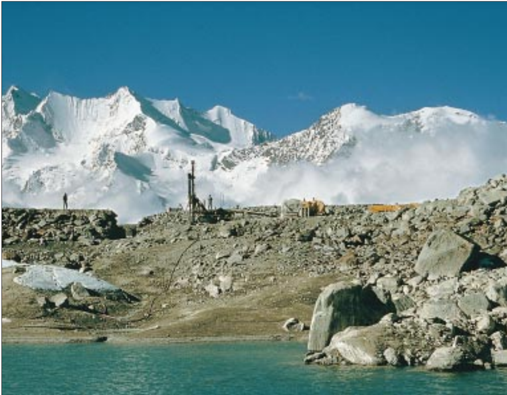
Photo 6.3: The injection drillings on the dam at Lake 1 protect the moraine against further erosion and prevent an outburst of this lowest-laying lake. The Dom and Lenzspitze mountains are in the background. (Photo: A. Kääh, University of Zurich)
