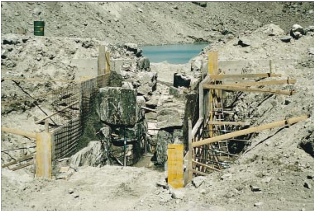
Photo 6.4: The overflow construction at Lake 1. The potential holding capacity of the lake is increased by lowering the level of overflow. This is necessary in order to catch a possible outburst of one of the upper lakes. (Photo: A. Kääb, University of Zurich)
